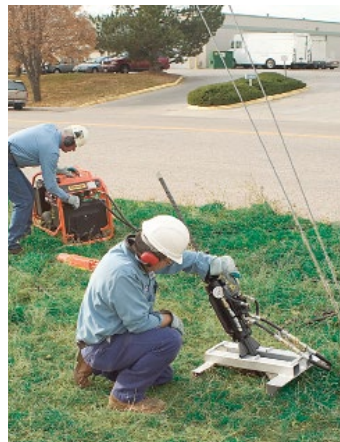
5. The portable power source operates the Load Locker which grips the adapter setting bar and rotates the anchor underground into position. The desired holding capacity is set with the Load Locker gauge.
