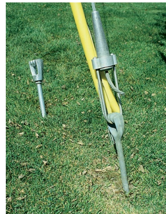
6. After removing the Load Locker, the eye is threaded to the end of the anchor rod. Now it's ready for guying.
