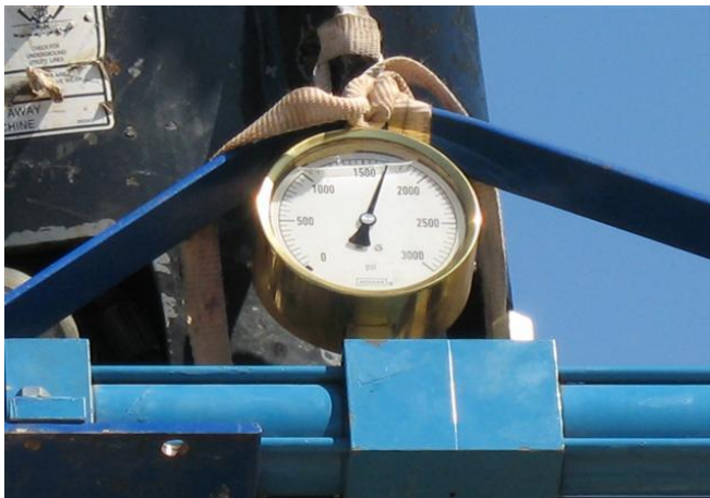
Typical calibrated hydraulic gauge and converted to torque used to measuring installing torque.
